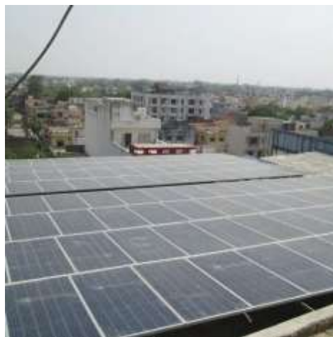
Figure 7.10: Solar Rooftop for Renewable Energy Integration
